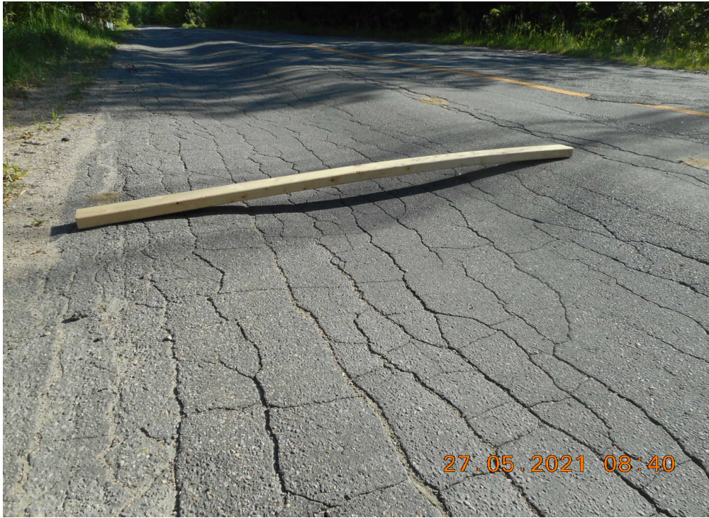
Figure 9: Wheel Track Rutting on Kilworthy Road (Section 1499)
